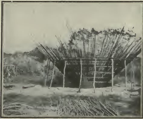
A ROOF FOR A HUT—WHEN COMPLETED, IT IS PICKED UP, TURNED OVER AND SET ON THE WALL
